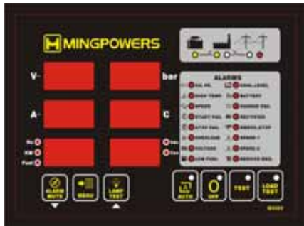
Control module Turkey Datakom 507
